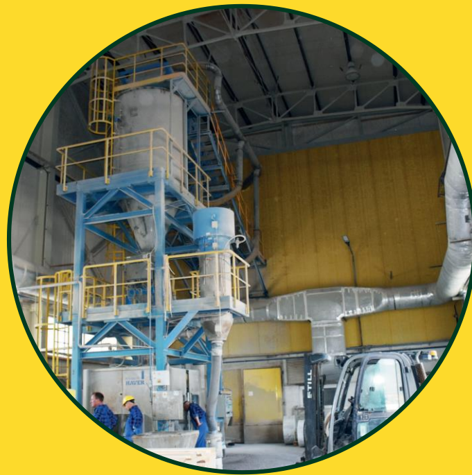
Completion of fertilizer packing units
