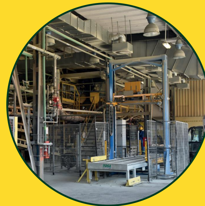
Installation of a second big-bag packing unit
